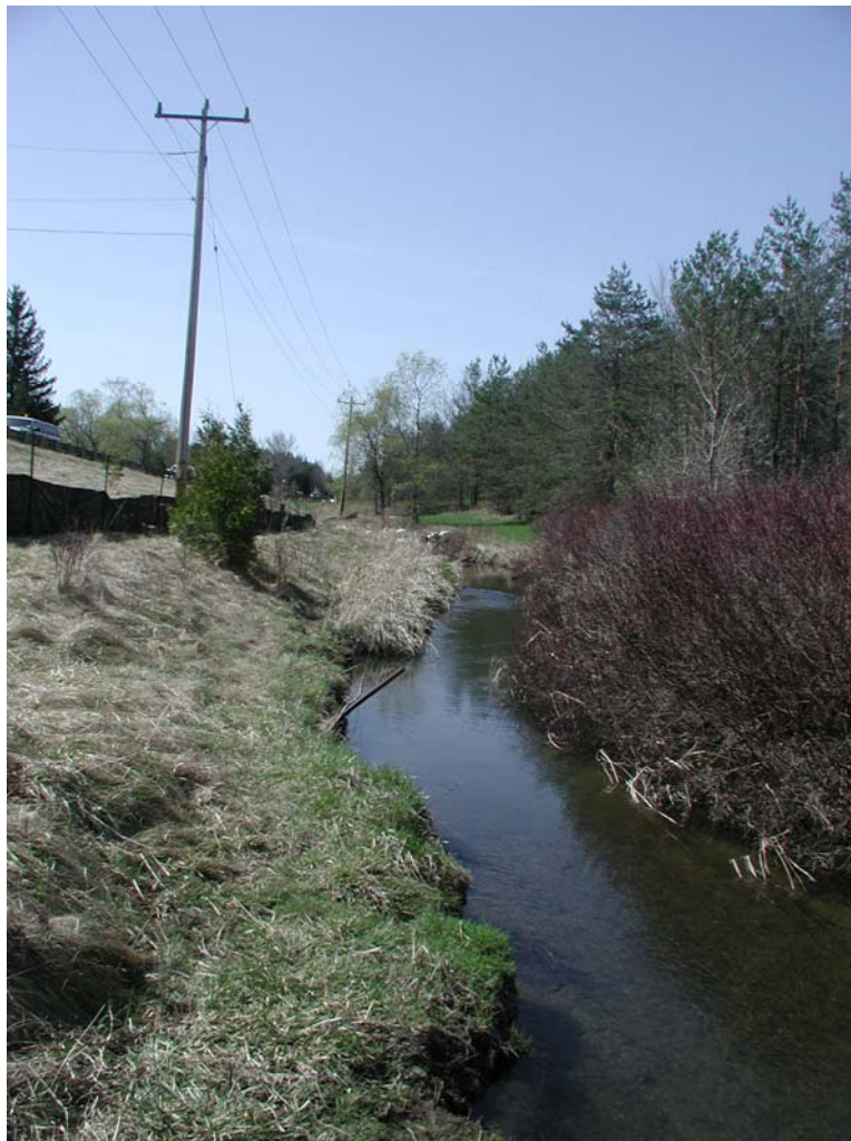
Figure 3 – Cold Water fisheries installation Spring of 2010 – looking east to west – 500mm HDPE
